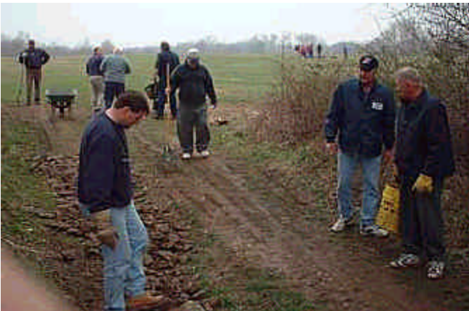
Al Tamburro supervises the placement of the rocks in the approach road gully
